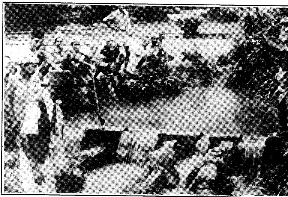
Figure 4. A saacho installed to distribute the flow from a main canal into four secondary canals according to the water allocation of each.
